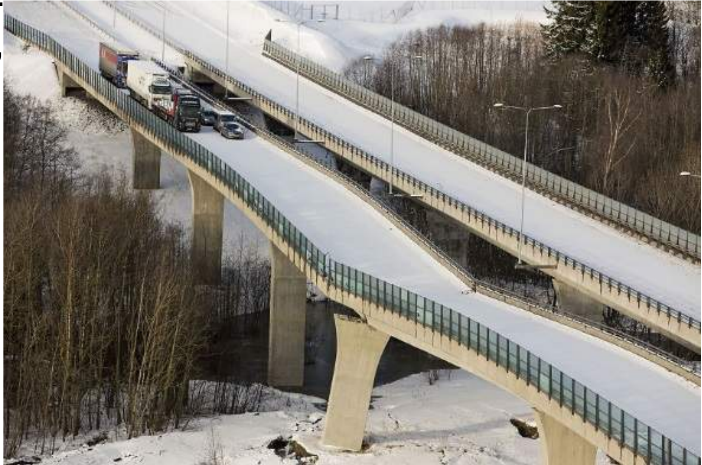
E18 expressway in Norway, February 2015 Slide in quick clay causing bridge collapse
